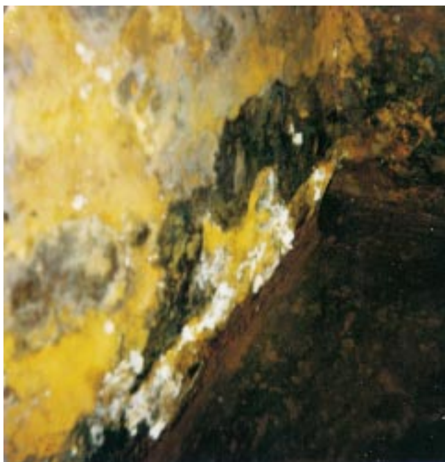
Figure 6.3 Ballast tank corrosion by SRB due to fish oil protection coating before cleaning
